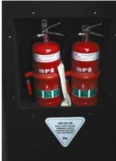
Fire safety gear at the ready
